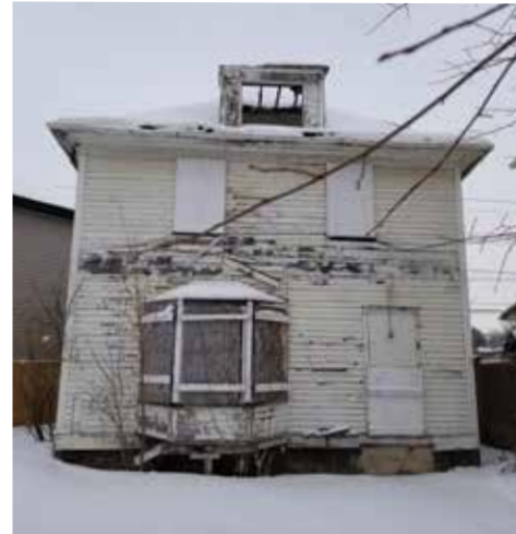
Before a demolition coordinated by DARC in Parkdale. Supplied by the City of Edmonton
